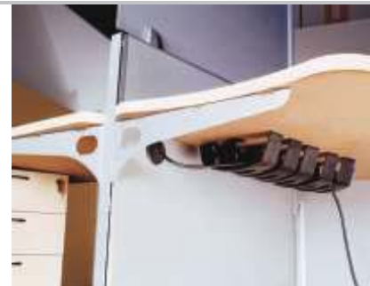
Panel to panel cable management
